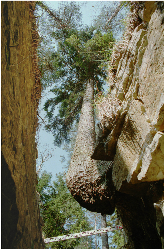
Figure 3: View from the crack to the sample tree 01 at site 01
